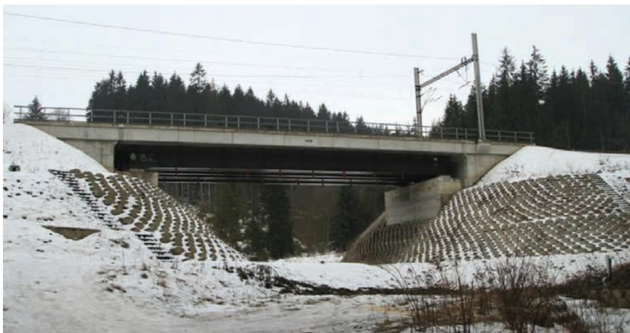
Fig. 20 Underpass constructed on the railway in the Mosty u Jablunkova city area close to the national border. GPS: 49°32'29.3"N 18°44'50.7"E- © Ivo Dostál
