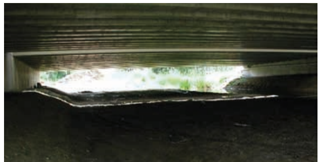
Fig. 36 Poorly implemented, too low wildlife underpass in Hungary 128 .
