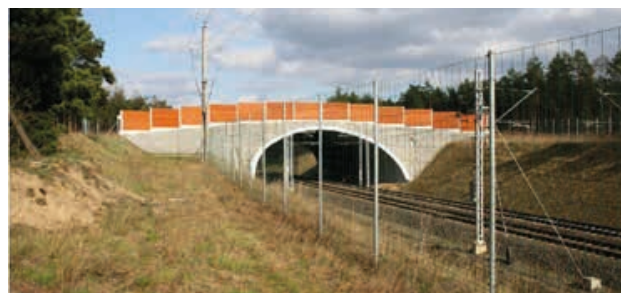
Fig. 24 In 2007, two upper transitions were created over the E20 railway line in Poland, section: Rzepin-Kunowice 119
