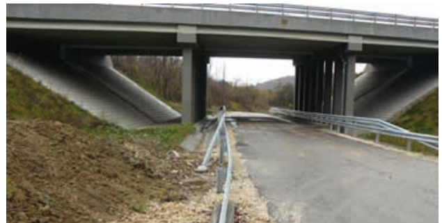
Fig. 35 Poorly implemented wildlife crossing with concrete on M7 Motorway at Kőröshegy in Hungary. GPS: 46°48'58.7"N 17°54'10.1"E 128
