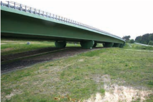
Fig. 37 S-3 expressway Międzyrzecz – Świebodzin. Viaduct for large animals close to Nietoperek in Poland, where the height is limiting the possibilities of the animals to move from one way to another.
